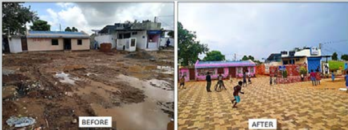
Open space development and community toilet restoration at slum Ishaneswara in Bhubaneswar Municipal Corporation
